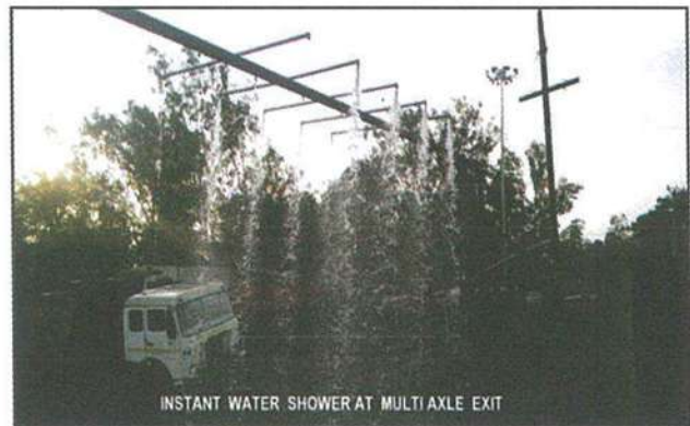
Instant Shower System at Hingula
